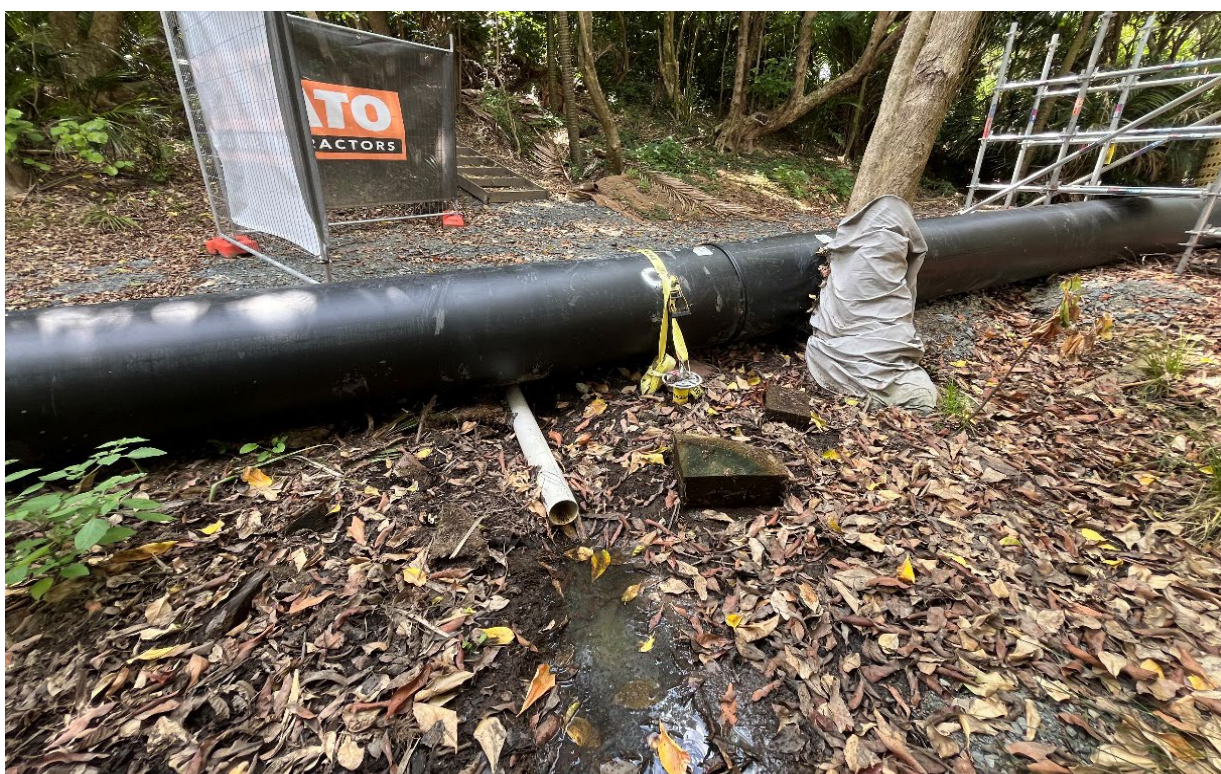
Figure 5: Culvert redirecting overland flow under the temporary accessway.
