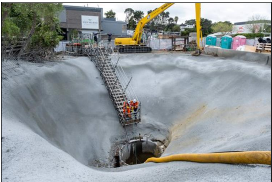
Figure 6: Ōrākei Main Sewer stabilised sink hole.
