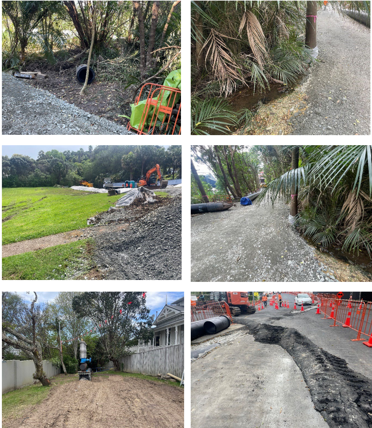
Figure 1: Photo schedule of erosion and sediment control works required.
